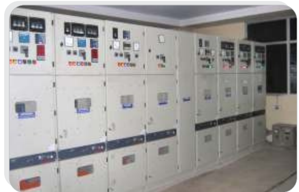
11kV VCB Panel
